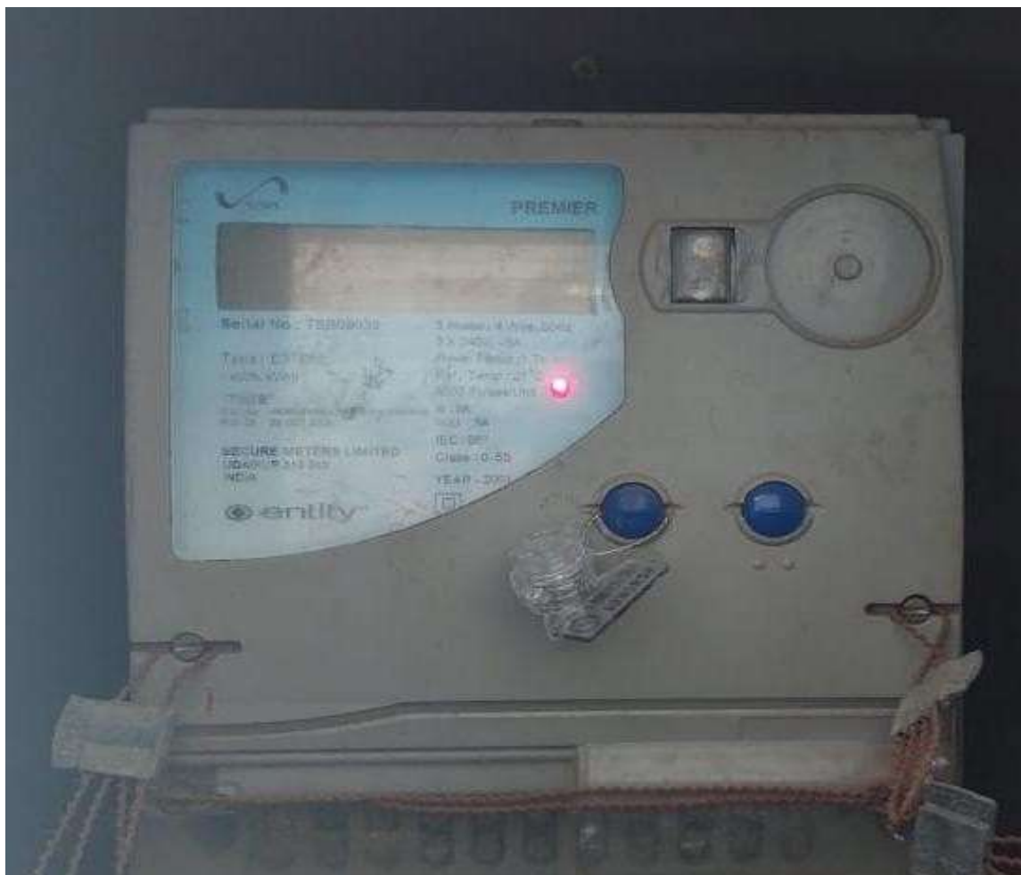
EB meter 110 kW
