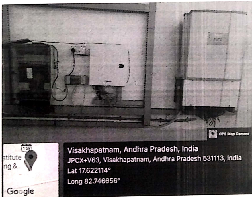
1) c) Meter for Solar energy system
