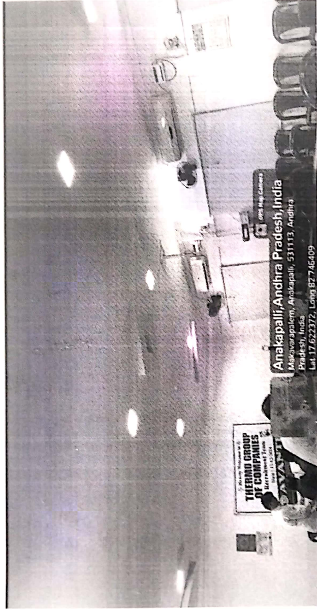
5) LED Lights installed in conference room
